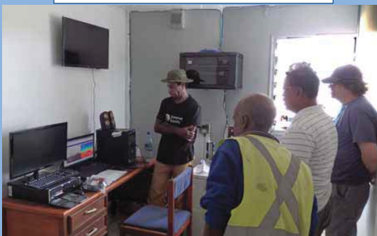
Installation at Tanna Airport Meteo
