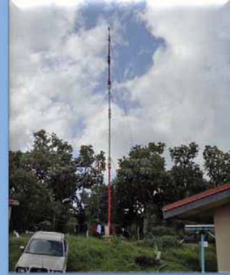
18m Tower @Health Centre
